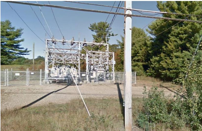
Eversource Substation on Oak Hill Road
