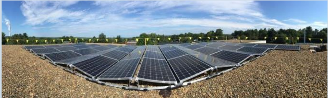
SOLAR PANELS INSTALLED AT PEMBROKE ACADEMY
