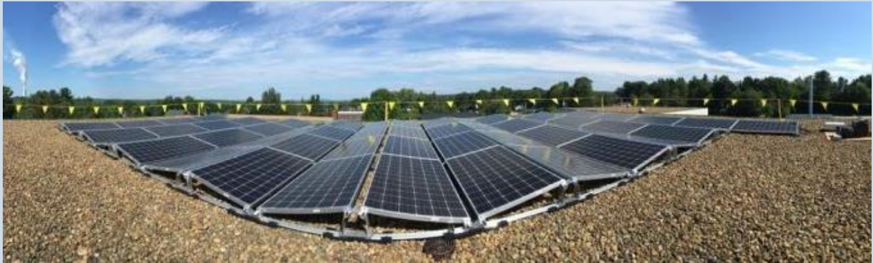
SOLAR PANELS INSTALLED AT PEMBROKE ACADEMY
